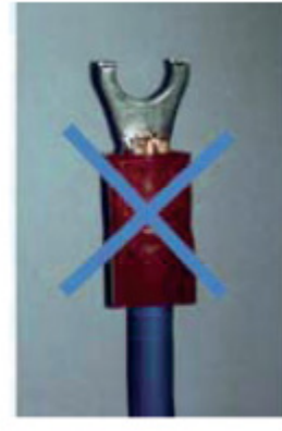
Terminal has been cut.
